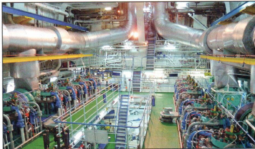
Superb maintenance keeps the Cegielski Sulzer workhorse power-plant smoothly running.
